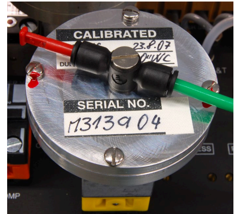
Figure 10 PE or MiniPurge® system pressure test point
